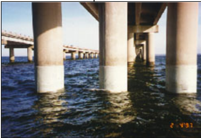
Cylinder Piles, Three per pier (1969) on right, two per pier (1956) on left.
